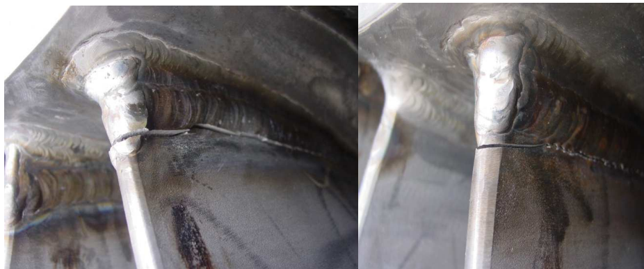
Figure 3: Photographs showing typical cracks evident at several short blade location, showing residual tensile stress
