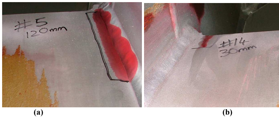
Figure 12: Dye penetrant on blades showing (a) long crack and (b) short crack types
