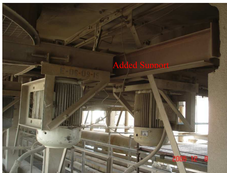
Figure 1. Motor End of Fan with Vertical Support Added Previously.
