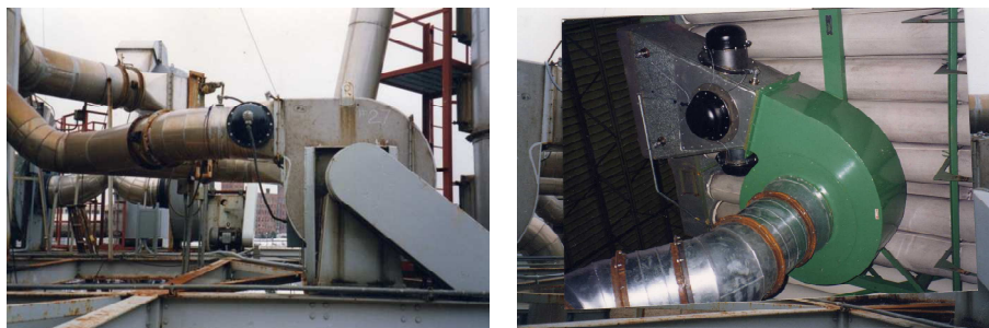
Figure 4 – ANC speakers located adjacent to fan discharge
