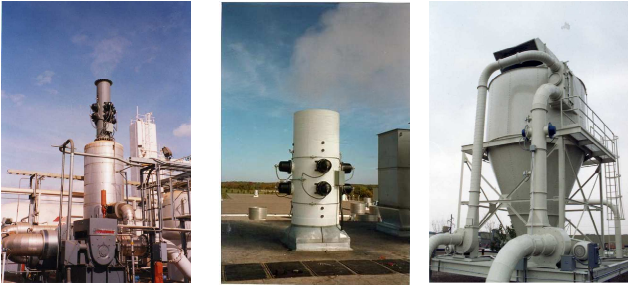
Figure 3-Various industrial fan ANC installations.
