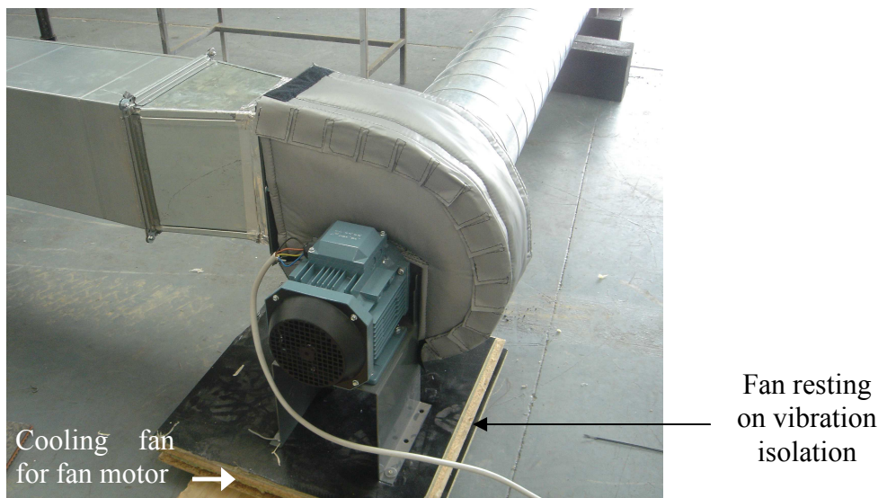
Figure 5: Acoustic jacket on scroll casing of the fan
