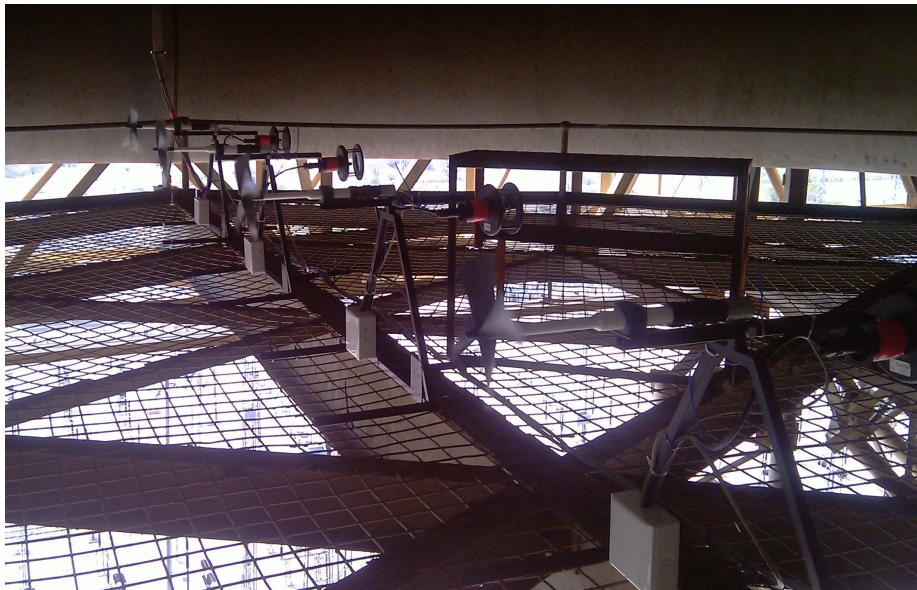
Figure 7: Frames placed at fan inlet
