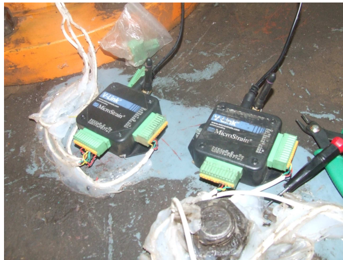
Figure 9: MicroStrain V-Link units attached to fan hub
